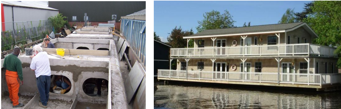
Figure 28: Construction of a Concrete Pontoon and floating ferro-cement structure along the river Thames. Source AquaBase.
