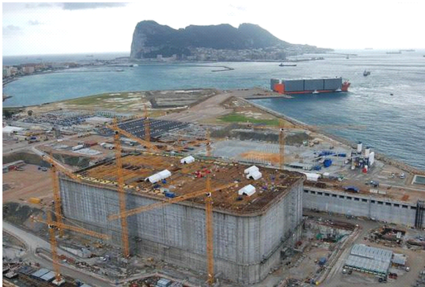
Figure 133: Construction of a concrete box for the LNG terminal “Adriatic” in Algeciras. Source: Acciona.
